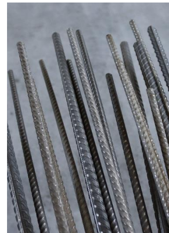
Ripped re-bar in sprayed mortar
